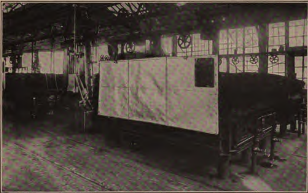
Fire Shield in Front of each Furnace in Heat-Treat Department
