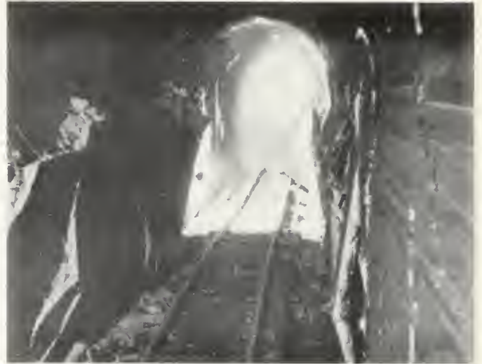
FIGURE 9. Cracked and buckled walls in tunnel 5. Camera is on the cave-in at 833 feet from the west portal; looking toward the cave-in at 632 feet. The tracks are bowed up about 1½ feet.
