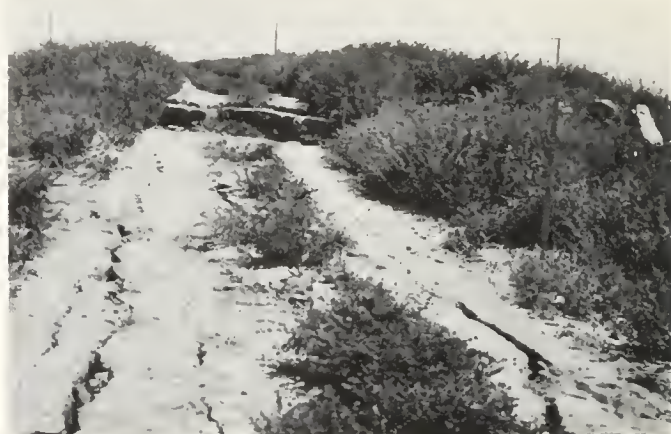
FIGURE 4. Buena Vista dam, east levee; view south. Subsidence and cracking of the fill caused by earthquake. Maximum settlement shown in photo is 2 feet. Photo courtesy California Division of Water Resources.
