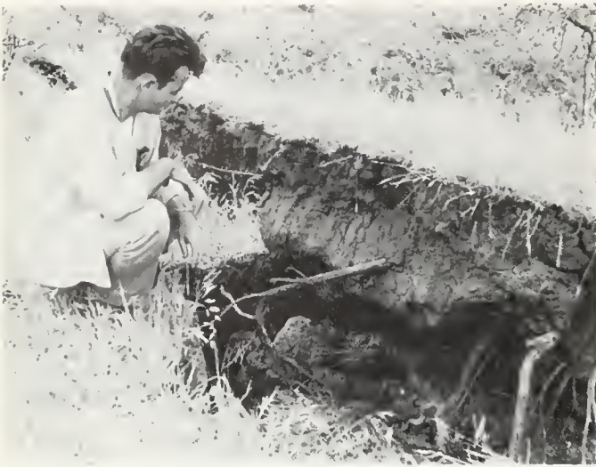
FIGURE 8. View west toward fault trace just east of south portal of tunnel 4. T. R. Fahy photo.
