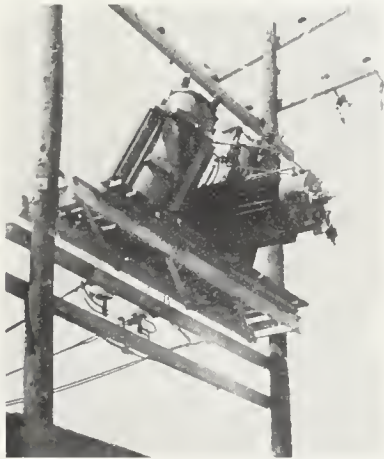
FIGURE 4. Damage to platform-mounted pole transformers. Long way of structure east-west. Photo courtesy Pacific Gas and Electric Company.
