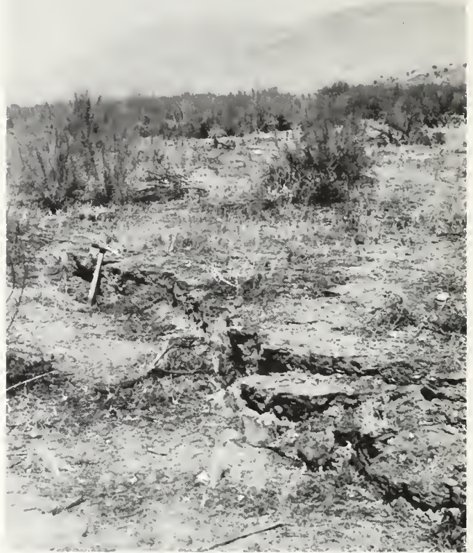
FIGURE 7. Cracks and scarplets in White Wolf fault zone, Tejon Hills, just northeast of Comanche Creek. Photo by Gordon B. Oakeshott.
