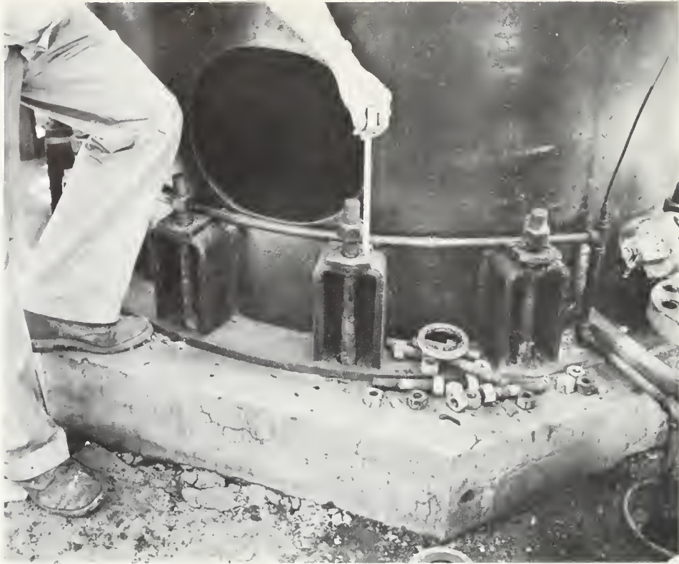
FIGURE 8. These thick steel bolts were stretched 1\frac{1}{2} inches as the tall 100-ton absorber rocked back and forth on its concrete base during the quake of July 21, 1952.
