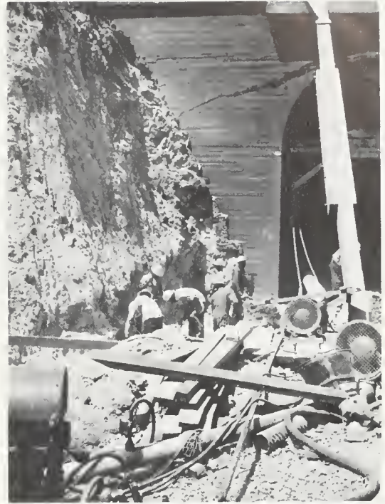
FIGURE 16. Excavating for footings and reconstruction of west portal of Tunnel 5, left side, August 5, 1952.
