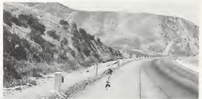
FIGURE 17. Cracking on upper side of fill, Highway 99, north of Grapevine station. Continued slumping in this filled section long delayed permanent repairs.
