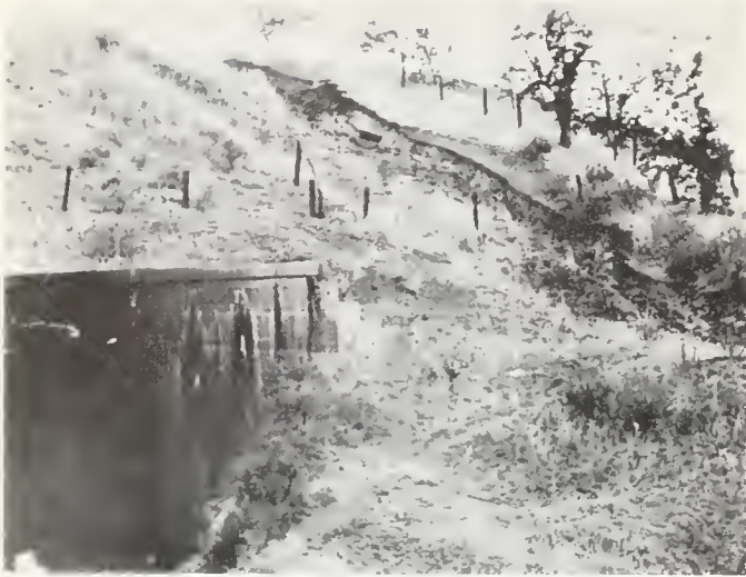
FIGURE 8. Surface expression of the normal fault shown in figure 7. The fault was traced several hundred feet to the right of the area shown in the photograph. View north.
