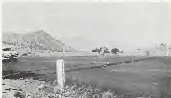
FIGURE 2. Transverse cracking on Highway 466 resulting from slumping of fill about a quarter of a mile west of trace of White Wolf fault.
