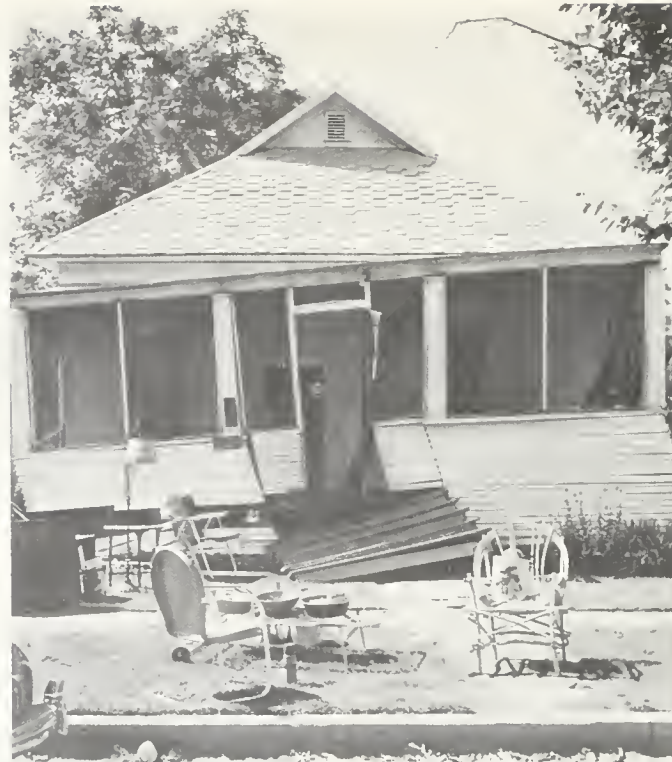
FIGURE 9. Frame house in Bakersfield after the earthquake of August 22, 1952. Photo courtesy The San Francisco Examiner .
