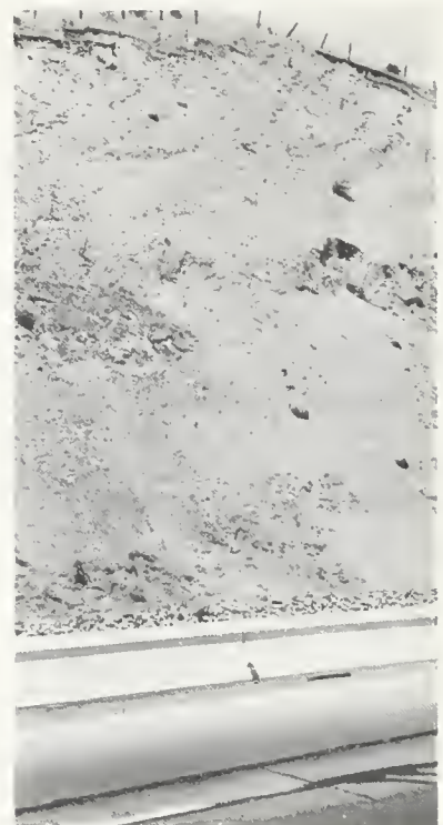
FIGURE 16. Sloughing and slumping on cut slope, Highway 99, near Grapevine.
