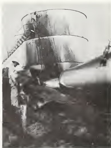
FIGURE 3. This storage tank was one of a battery of three. It collapsed, spilling 800 barrels of oil, but the two adjacent tanks were relatively undamaged.
