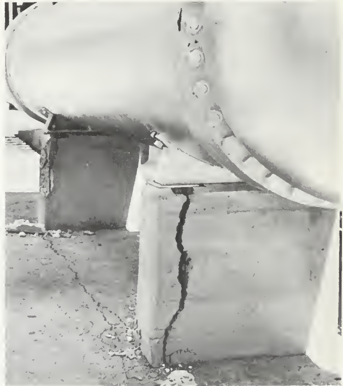
FIGURE 9. A strong westerly component of movement is indicated by the slippage of this tank along its fractured concrete base. A similar direction of movement was noticed in other storage tanks throughout the San Joaquin Valley.
