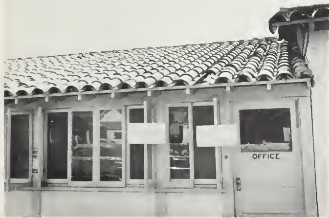
FIGURE 9. Detail of building shown in figure 8. Slight damage—one roof tile shaken off, stucco finish cracked.
