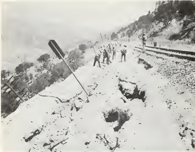
FIGURE 18. Broken fill between Tunnels 6 and 7.
