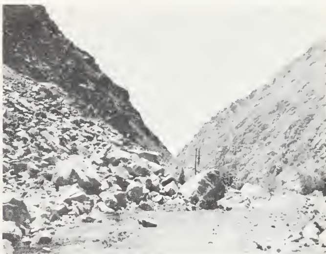
FIGURE 22. Main rock slide of granitic fragments closing Kern Canyon road (Route 178) after July 21 earthquake.
