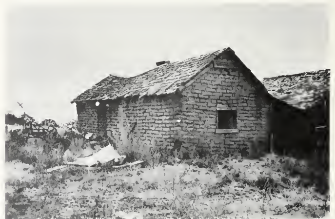
FIGURE 14. Adobe construction on a few inches of fill overlying rock. Undamaged building on south side of Cummings Valley. Building is very old; cracks are not due to earthquake but are old cracks with edges rounded by rainwash.
