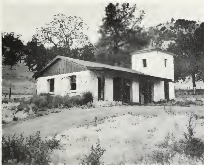
FIGURE 15. Part adobe, part frame construction on approximately 10 feet of fill. Damaged building on northwest side of Cummings Valley. Adobe wall is cracked, but frame portion of building is intact.
