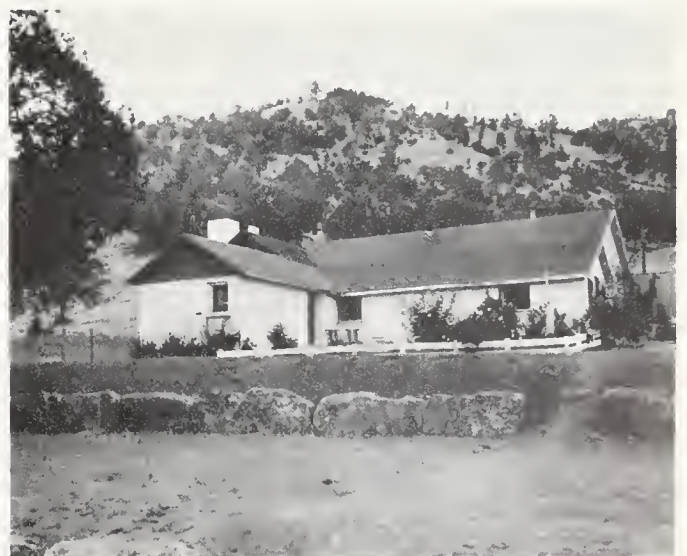
FIGURE 18. Adobe and frame construction on approximately 10 feet of fill overlying rock. Slightly damaged building on northwest side of Cummings Valley. Adobe portion of building is cracked; frame portion is undamaged.
