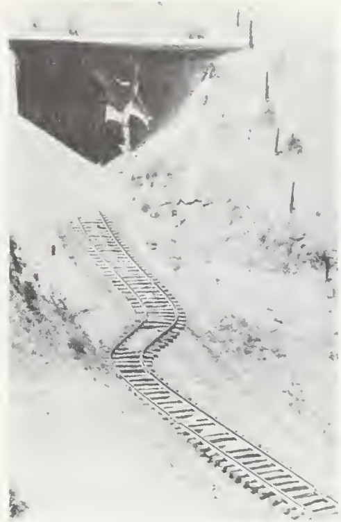
FIGURE 6. Sharp bend in the tracks south of tunnel 3 strikingly demonstrates that the ground had been shortened in this area. A landslide blocks the east portion of tunnel 3.
