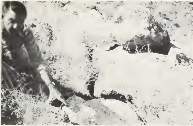
FIGURE 27. Landslide cracks on slopes above Kern Canyon road. These allow entry of storm water and bring constantly renewed slides and rock falls.
