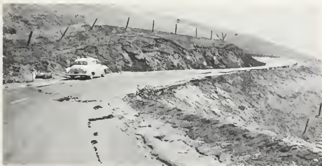
FIGURE 10. Damage to pavement on State Route 140, White Wolf grade. This highway roughly parallels the White Wolf fault for several miles.
