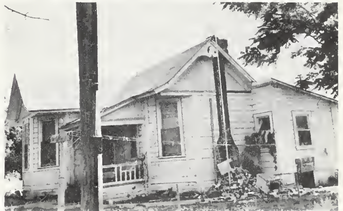
FIGURE 17. Frame construction on alluvium. Damaged dwelling in residential district of Tehachapi. Frame portion only slightly damaged; brick chimney pulled away from frame.
