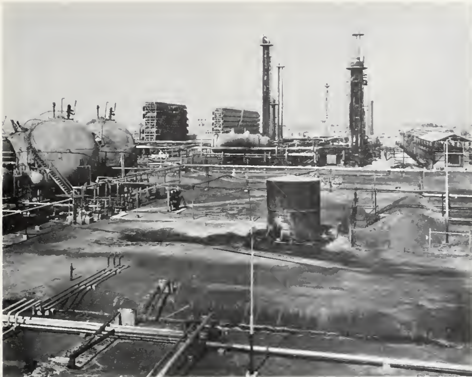
FIGURE 6. A general view of the Paloma cycling plant showing the blackened area of explosion and fire. The spherical butane storage tanks are at the left, remaining cooling towers and tall vessels in the center, and compressor plant at the extreme upper right.
