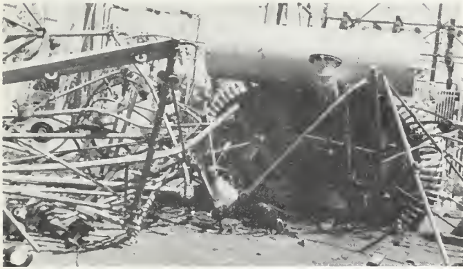
FIGURE 3. Detail of transformer damage at Weedpatch substation. View north. Photo courtesy Pacific Gas and Electric Company.
