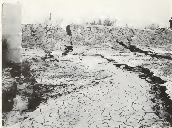
FIGURE 3. Northwest-trending cracks 1 mile west of U. S. Highway 99 and 7.5 miles south of McKittrick Road. Note damage to farm reservoir. Cracks vary in direction; trend of those in photo N. 60° W. View southeast. Photo courtesy California Division of Water Resources.
