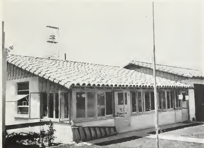
FIGURE 8. Reinforced concrete-block construction on alluvium. Slightly damaged building in Tehachapi.
