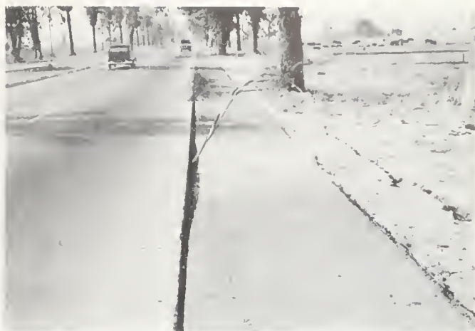
FIGURE 21. Settlement of shoulder surfacing amounting to maximum of 11 inches, east lane of U. S. 99, near Wheeler Ridge.
