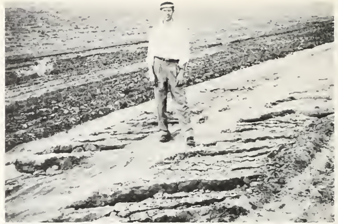
FIGURE 14. Fracturing along road marking south border of mapped field. Photo by E. M. Bien.
