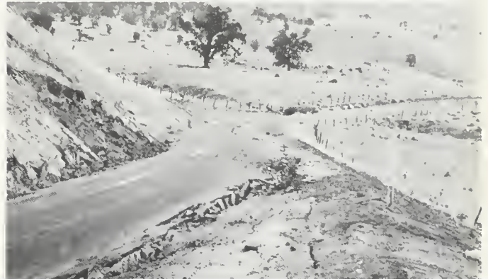
FIGURE 11. Marginal cracking in filled area, and minor landslide in cut slope. White Wolf fault at break in slope at top margin of photograph. View southwest along State Route 140.
