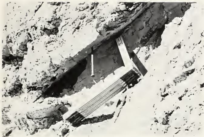
FIGURE 10. Fault and gouge in west side of railroad cut. Hanging-wall block (upper) probably moved upward during earthquake, but displaced nail heads show downward landslide-type movement following earthquake.
