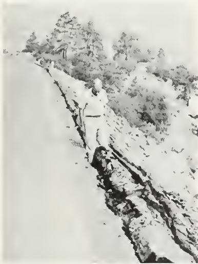
FIGURE 9. Marginal cracking in filled area of Highway 466, opened up in aftershocks.
