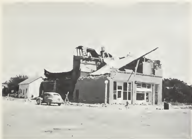
FIGURE 7. Brick construction on alluvium. Badly damaged building in business district of Tehachapi. Undamaged frame building at left.
