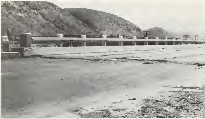
FIGURE 4. Bridge over Walker Basin Creek showing cracking resulting from settlement of fill at the approach.
