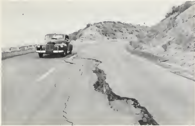
FIGURE 8. Cracks in pavement in filled area east of sand cut, Highway 466, opened up by severe aftershock of July 29, 1952.
