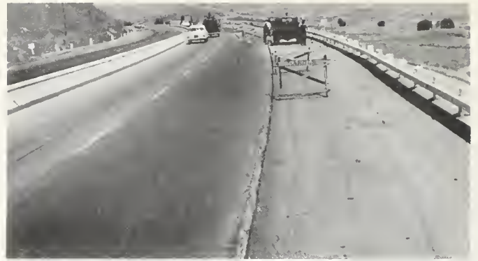
FIGURE 15. Shoulder settlement in fill, with a resulting step-off at edge of concrete pavement, U. S. 99, near Grapevine.
