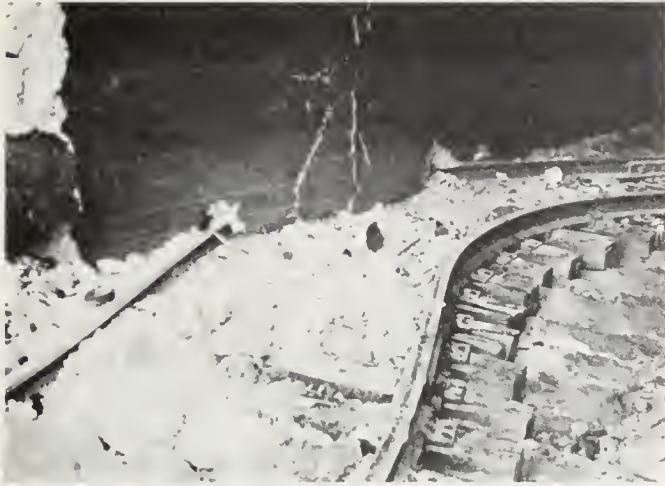
FIGURE 5. Damage near the east portal of tunnel 3. Apparently the wall was raised just as the track bent, and the wall then came down on top of the rail. View northwest.
