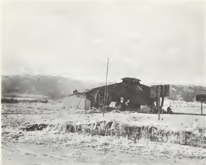
FIGURE 10. Improperly built concrete construction on thick alluvium. Damaged schoolhouse in Cummings Valley.
