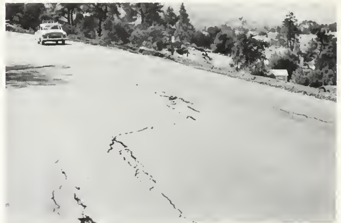
FIGURE 7. Transverse and longitudinal cracking of pavement in filled area, Highway 466.
