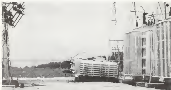
FIGURE 7. San Bernard substation, transformer damage. Photo courtesy Pacific Gas and Electric Company.
