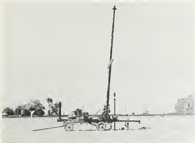
FIGURE 8. Dry rotary shot hole drill, Shell Oil Company, 1928. Photo supplied by Frank E. Vaughan.
