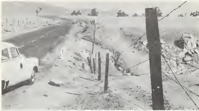
FIGURE 12. Erosion on margin of pavement, State Route 140, resulting from diversion and increased flow of minor stream after earthquake of July 21, 1952.
