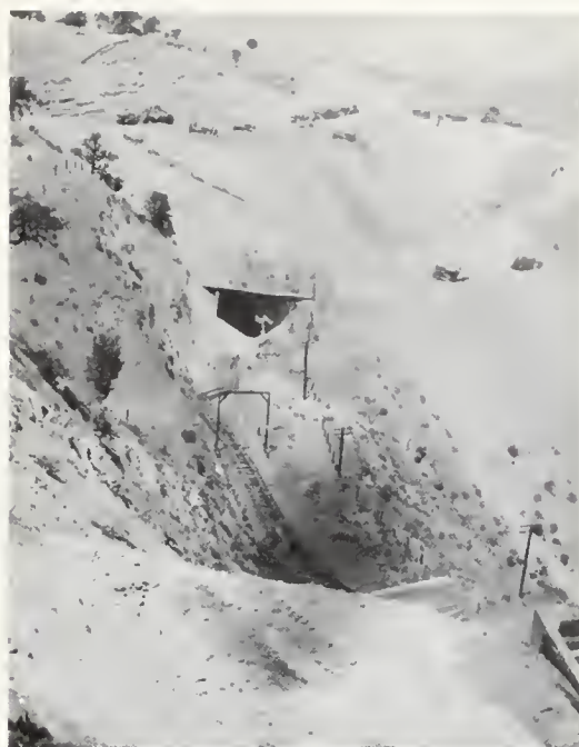
FIGURE 7. East portal of Tunnel 3 seen from top of Tunnel 4, showing daylighting in progress over Tunnel 3.
