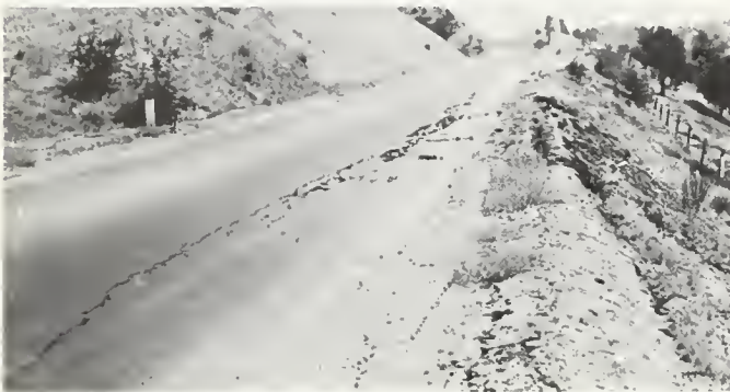
FIGURE 5. Cracks on Highway 466 resulting from settling of marginal fill.
