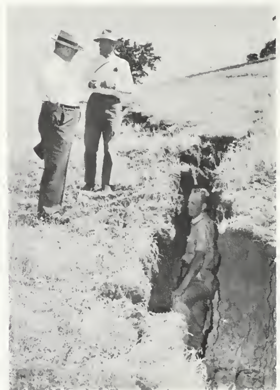
FIGURE 21. Crack in hill between Caliente and Tehachapi Creeks. Elevation approximately 3000 feet. August 9, 1952.
